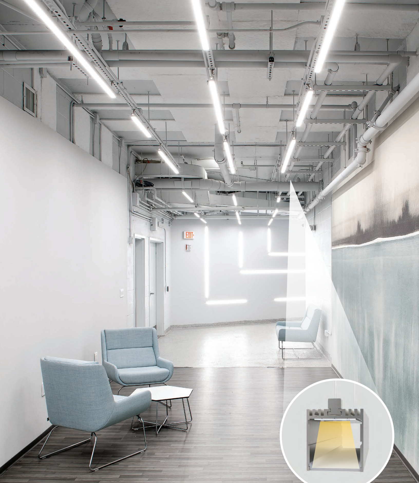
PrimaLine 4.4 Gen 2 Tape Light - 4200K Suspan 1 Channel Hallway - Jersey City, NJ
